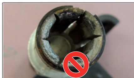
Fig. 46: Socket contact contaminated due to acid exposure
